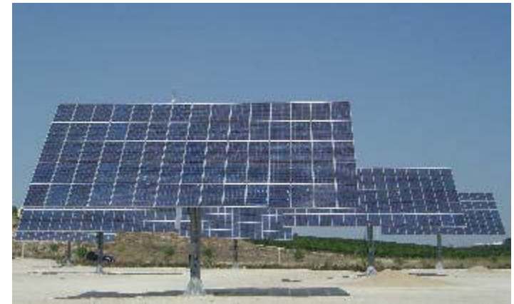
Murcia, Spain [RenewableEnergyAccess.com] A 5 MW solar tracking PV plant with a total surface exceeding 3.5 million sq. ft. using 500 2-axis solar trackers will be installed in Caravaca de la Cruz (population: 22,880) in Murcia, Spain by Soltec Energias Renovables.
